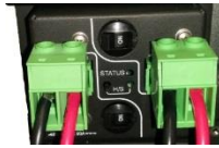
Figure 22: PEM's Circuit Breaker Position
